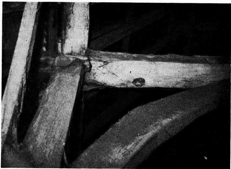
FIG. 1. The pre-dovetail method of assembling a transverse building frame, in the southern barn. The brace to the tiebeam is squint-lapped to the sides of both post and beam. Note the significant absence of the post-head jowl.
